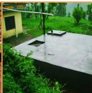
Rain Water Harvesting
